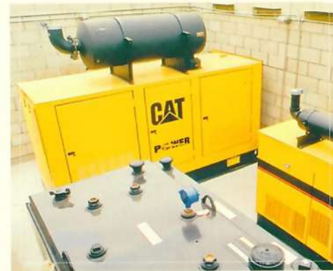
POWER BACKUP FOR GENERAL UTILITY
